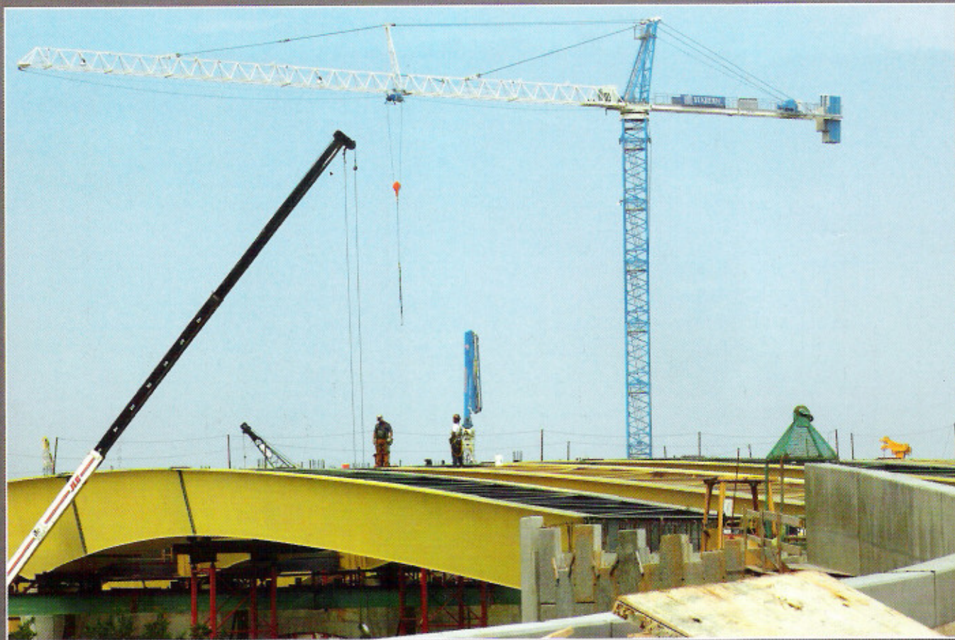
Steel workers install beams for the new 17th Street bridge over the I-75/85 Connector in Midtown Atlanta. The bridge is scheduled to open Dec. 31.
